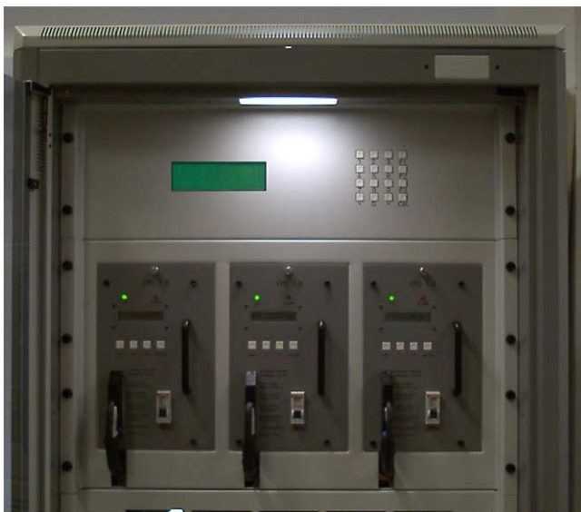
Fig. 17. Battery monitoring implemented on a telecommunication power system.
